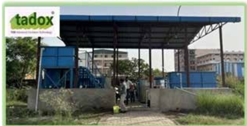
20 KLD TADOX® Plant in Textile CETP in Kanpur; Funded by National Mission for Clean Ganga, MoJS, GoI
